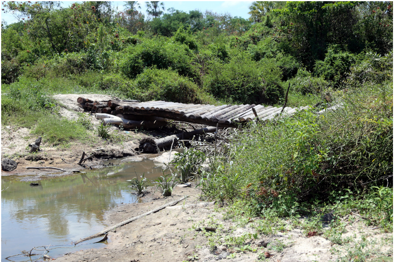
Fig. 2: The bridge did not seem suitable for us to drive our car over.
